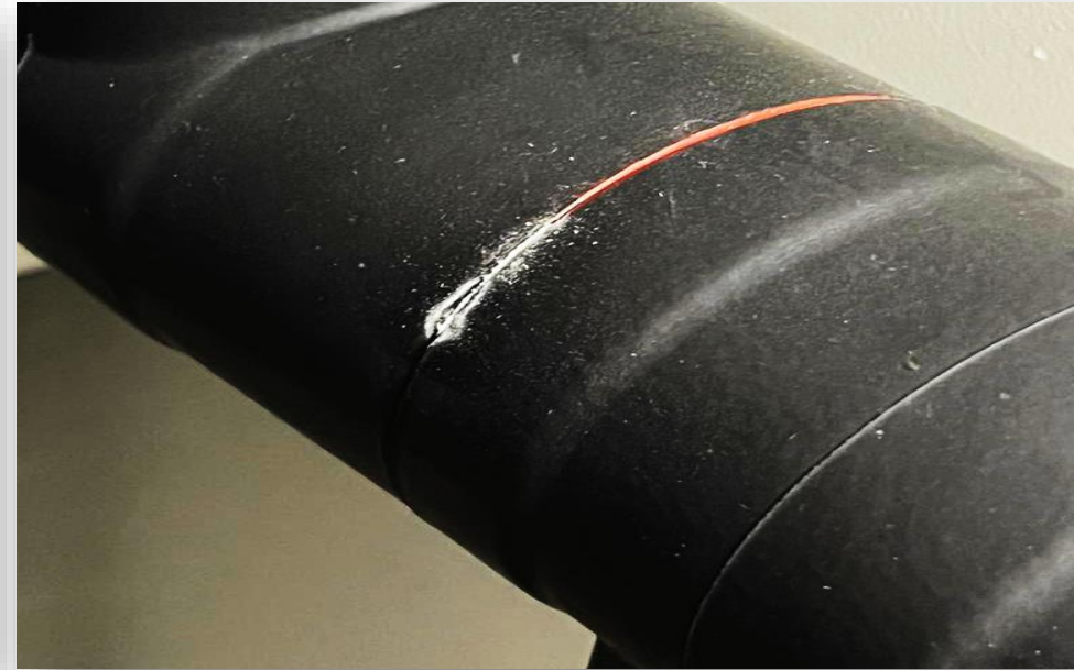
Visible cracks at Insulating body
